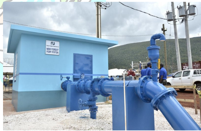
New Forest Pump Station
